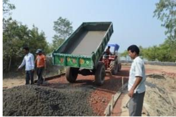
Human activities in the Sundarbans delta: Concrete Road and embankment building programme after Aila cyclone in 2009.
